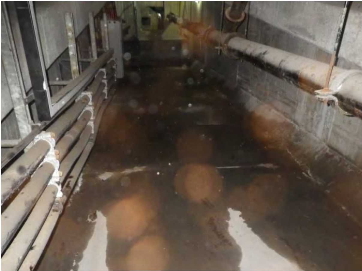
Photo 3: Water ingress from a duct in the southern half-joint
