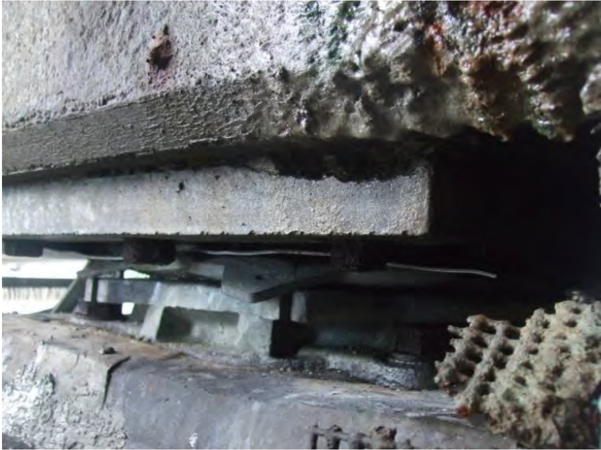
Photo 1: Cracked and broken top plate on bearing at south abutment
